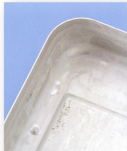
Figure 2: Corrosion of Anodised Aluminium
