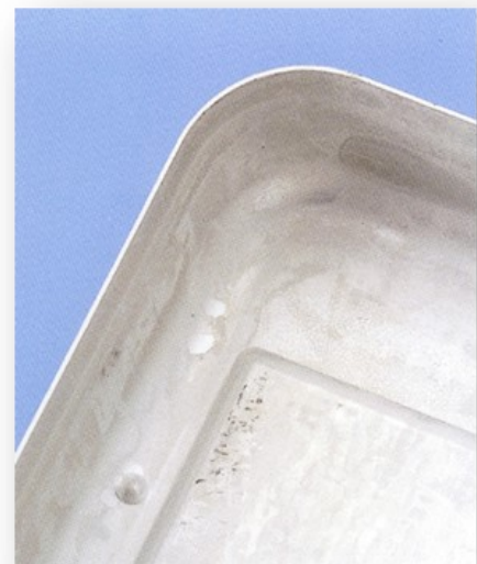
Figure 2: Corrosion of Anodised Aluminium
